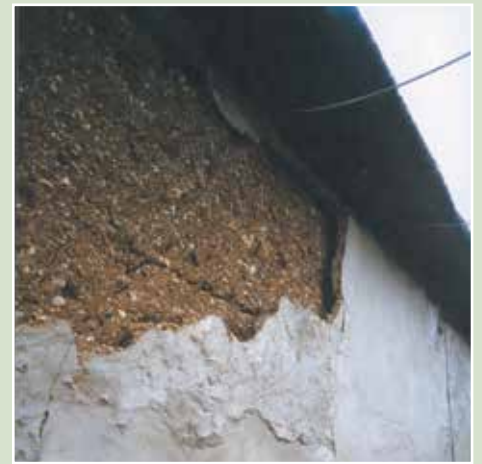
Moisture trapped behind cement render
