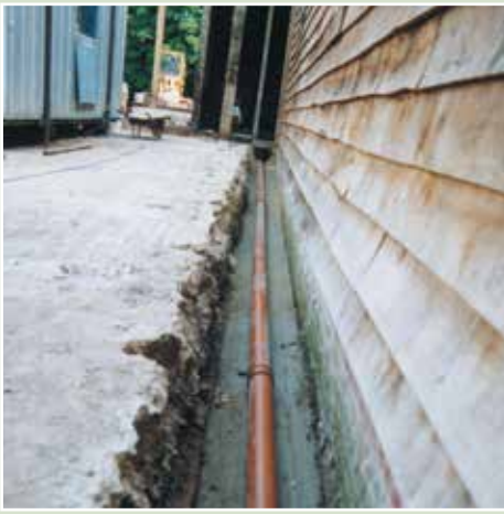
Creating a drainage channel to reduce ground water level against a wall.
