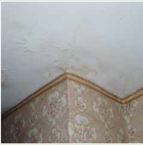
◀ Example of damp penetration
