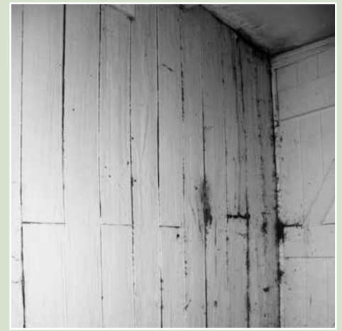
Moisture leading to damp ▶
